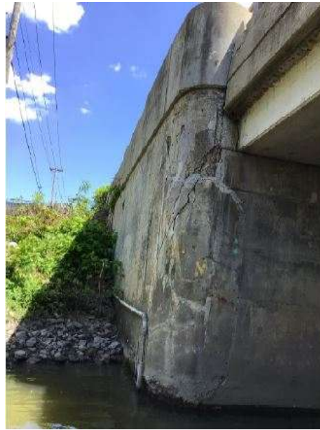
View of Exposed Rebar, Spalled & Delaminated Concrete, Failed Epoxy Repair and Map Cracking on Northeast Wingwall, Looking East
