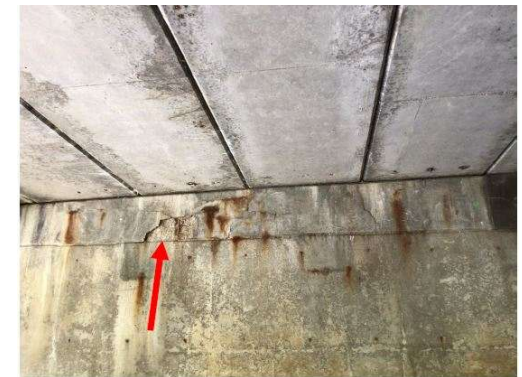
View of Delaminated, Cracked and Spalled Concrete with Exposed Rebar and Rust Staining on Pier 2, Looking West
